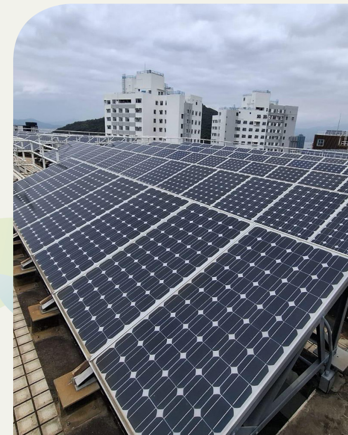
FIGURE 9: Solar Panel System in the Jockey Club Building for Interdisciplinary Research
